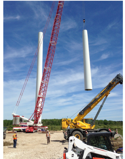
Skyway 8 Wind Farm, Ontario
